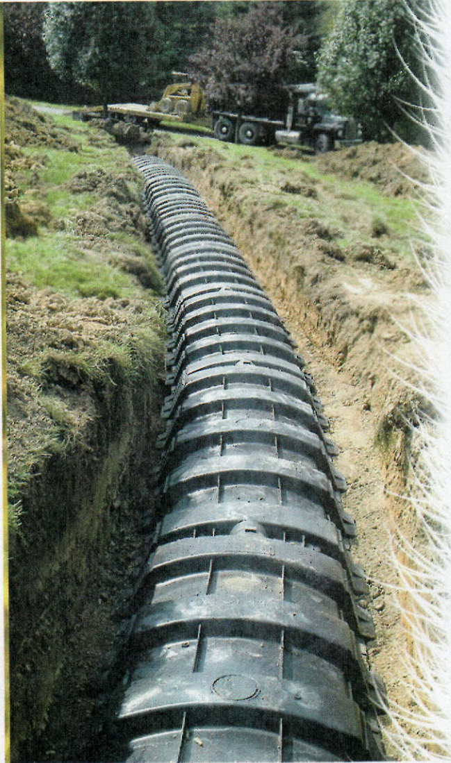
Alternating drainfields provide relief for a failing system. Here, a second drainfield is installed.
